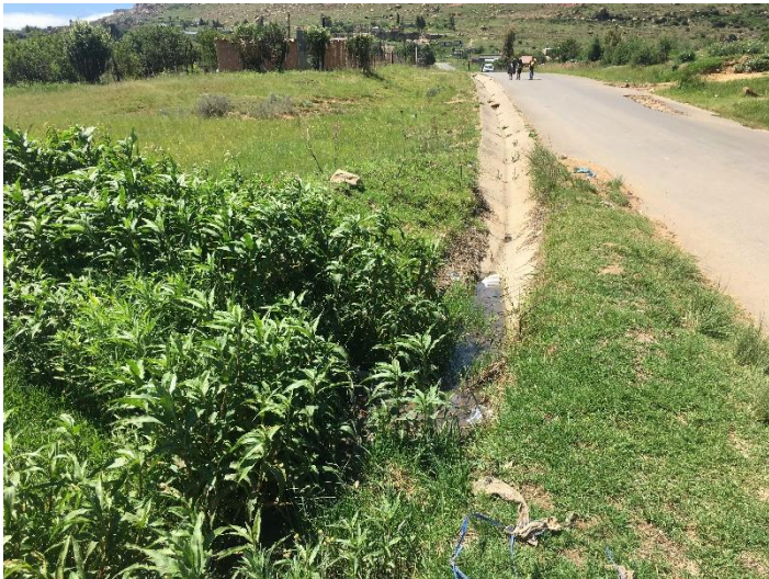
Figure 3: Existing Storm water infrastructure adjacent to the tarred road that is currently not maintained. (Direction – SE)
