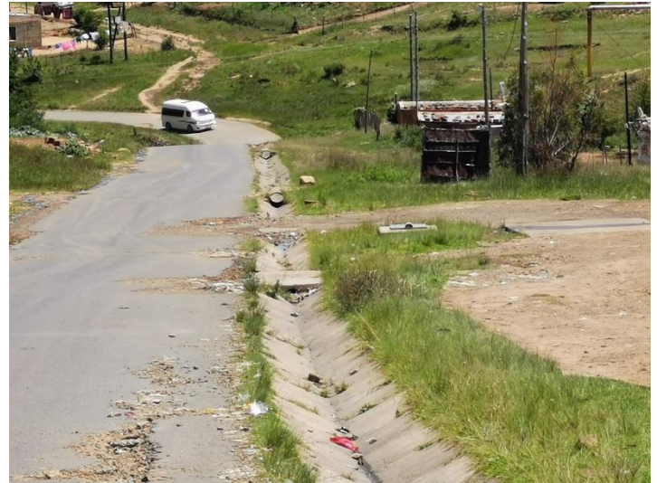
Figure 2: Existing stormwater drainage where the proposed discharged pipeline is to be located
