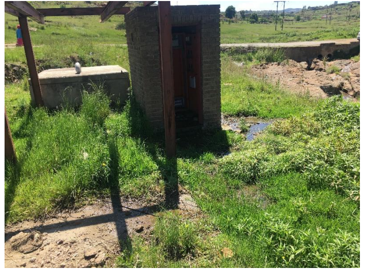
Figure 14: Dilapidated sewage pump station noted to be seeping raw sewage directly into the Metsi Matsho tributary
