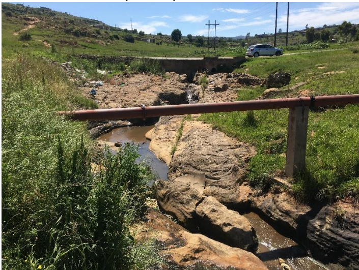
Figure 16: Water pipelines crossing the Metsi Matsho Tributary
