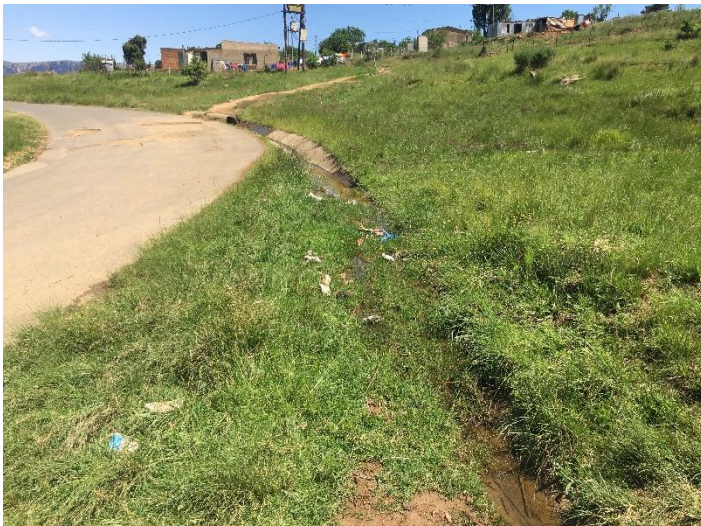
Figure 5: Existing and degraded Storm water infrastructure with overgrown vegetation (viewed from the south)
