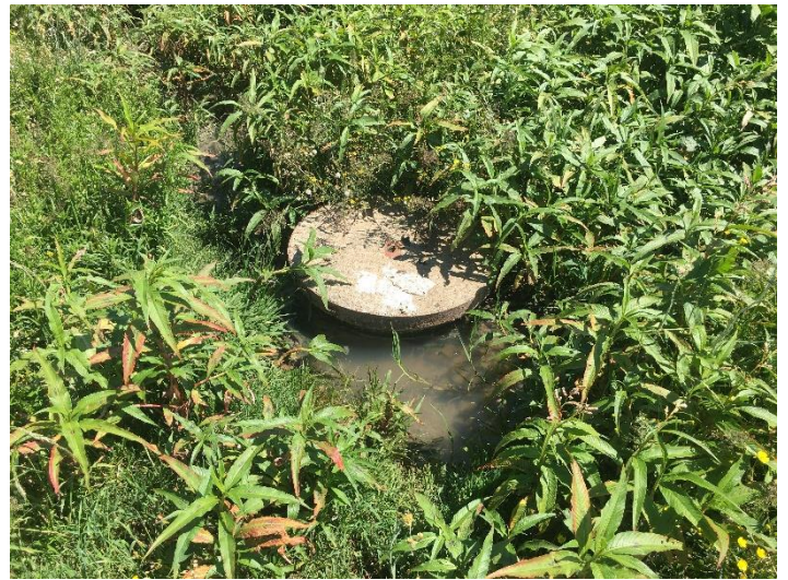
Figure 17: Manholes noted around site seeping sewage directly into the tributary
