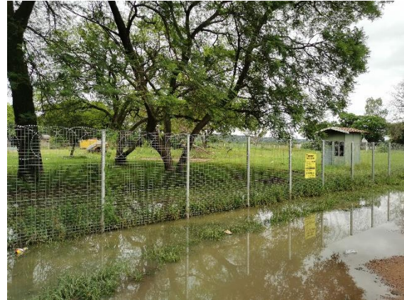
Figure 9: Road section with poor drainage
