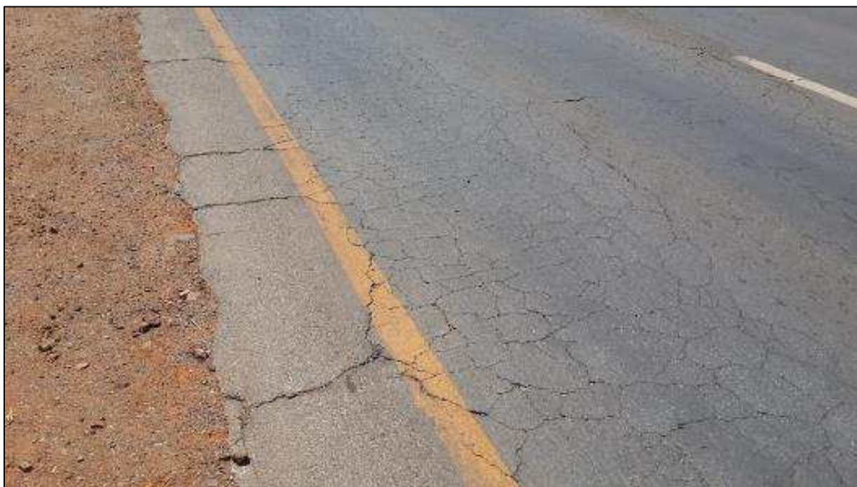
Photo 7.4: Typical crocodile cracks along the second section at km 4.00
