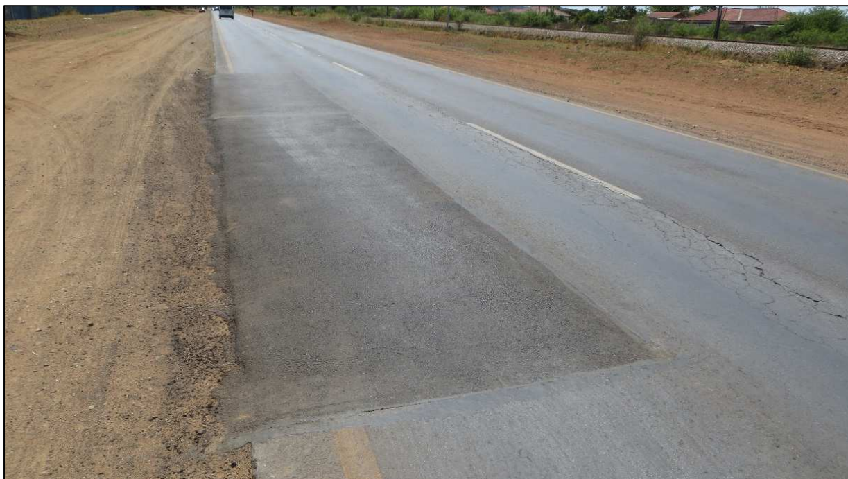
Photo 7.5: Patch, rut and crocodile cracks at km 2.40
