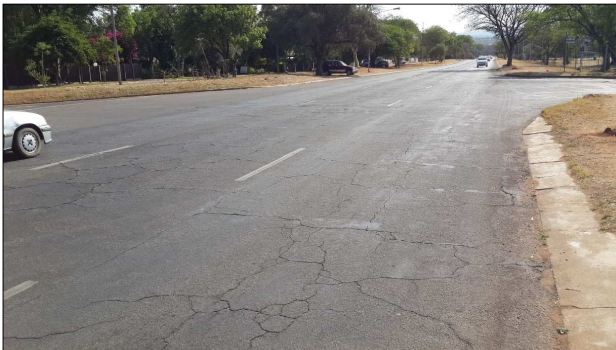
Photo 7.9: Typical appearance of section in Modimolle showing block and surface cracks
