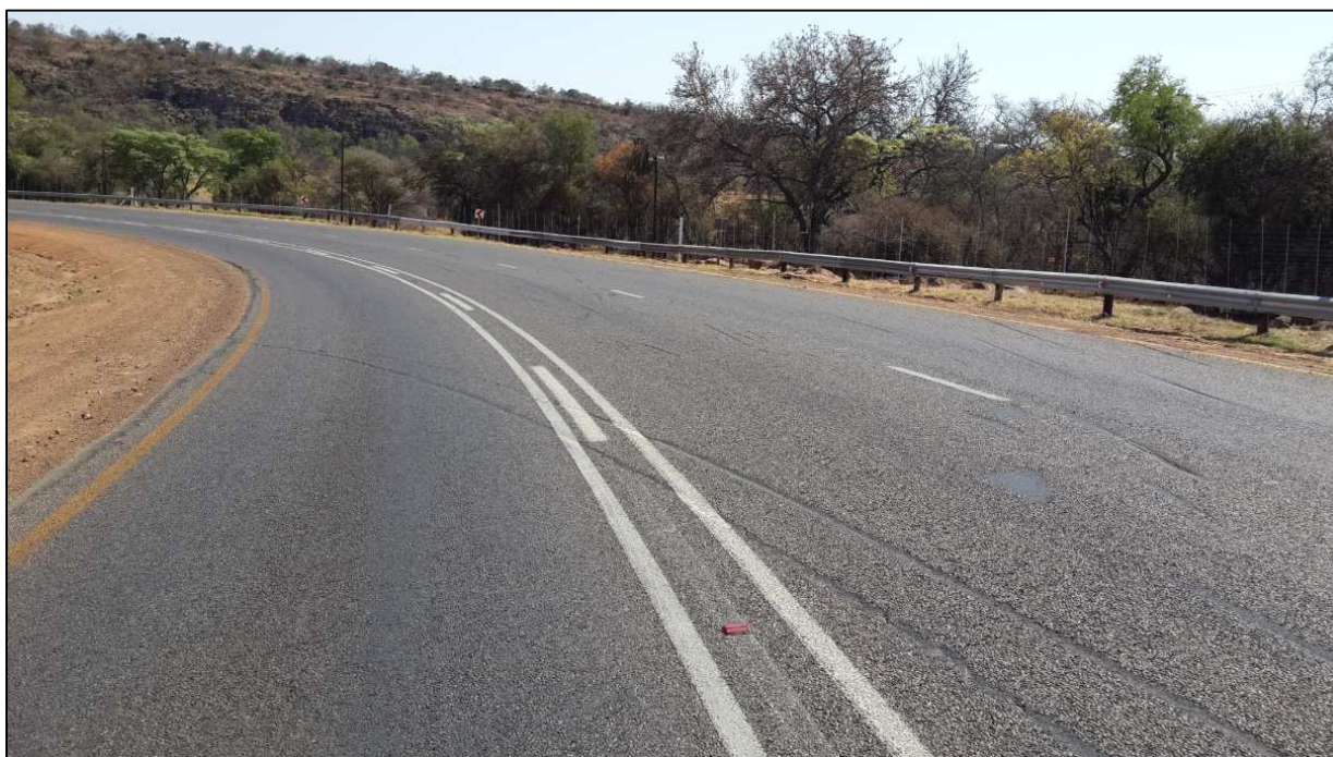
Photo 7.8: Mechanical damage on the curve at km 15.40
