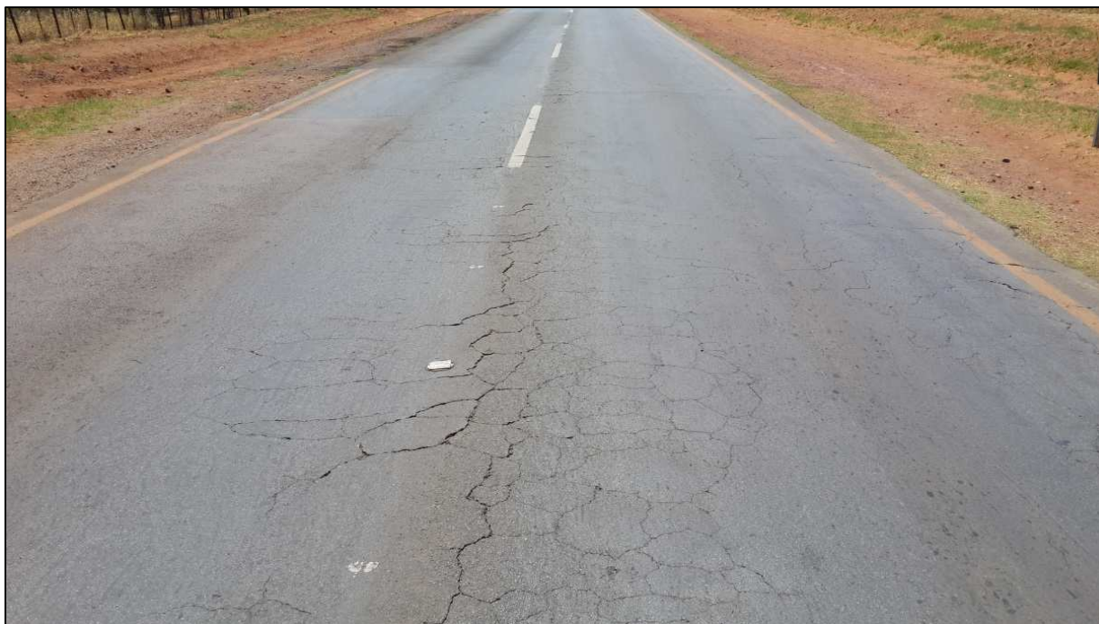
Photo 7.3: Rutting and typical appearance of the second section at km 4.60
