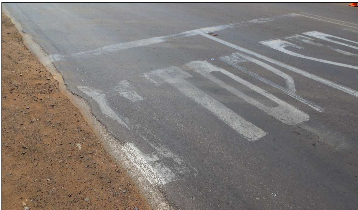
Photo 7.2: Shoving at Mile Street intersection (km 0.70)
