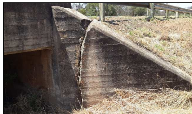
Figure 11.11: Cracked through wing wall
