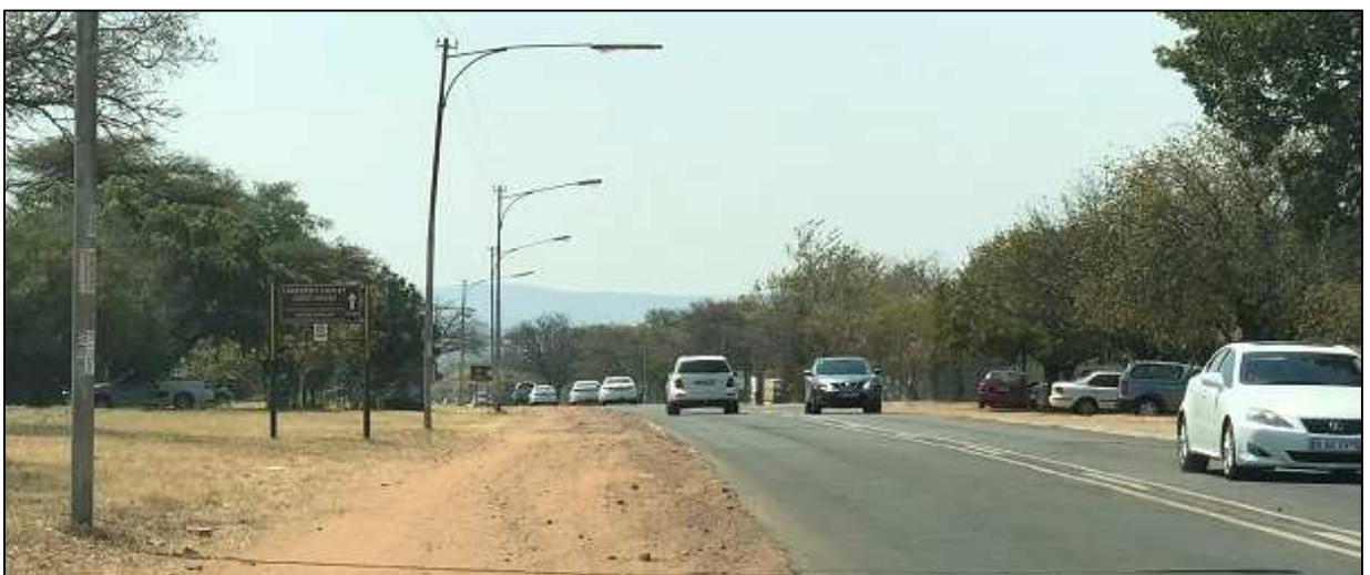
Photo 13.2: Two types of street light fittings installed in Modimolle on the Left hand side
