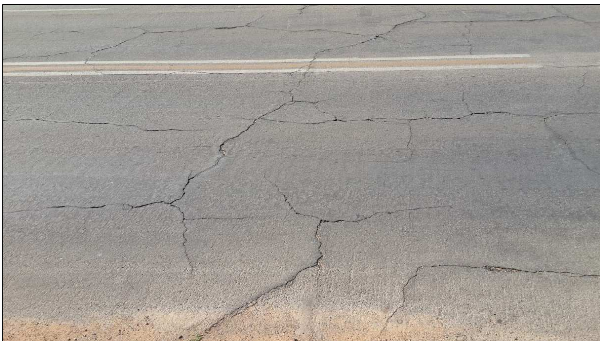
Photo 7.10: Block cracks from km 25.10 to km 26.80
