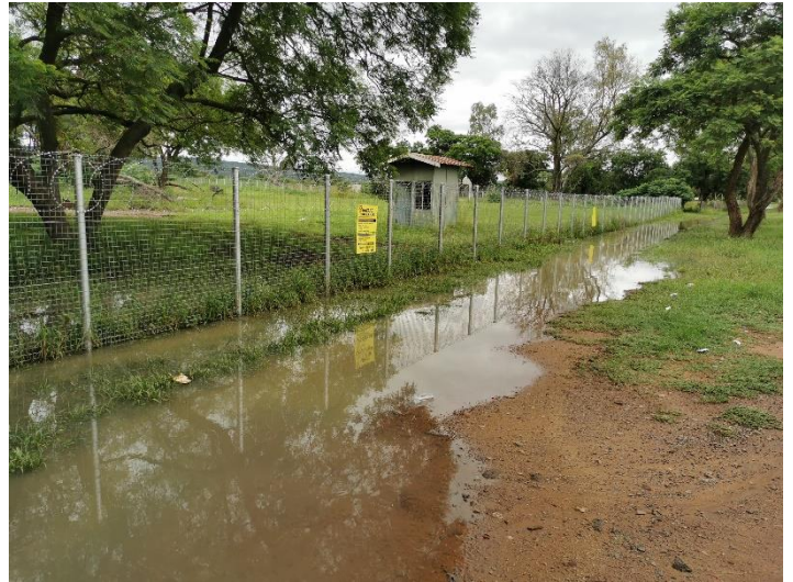
Road section with poor drainage between km 0.0 and km 1
