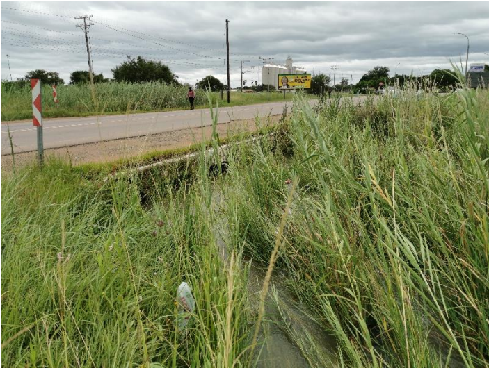
Major box culvert with insufficient drainage capacity
