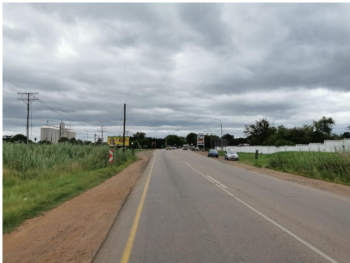
Pavement of National Road R101 Section 8 is generally in a fair to good condition
