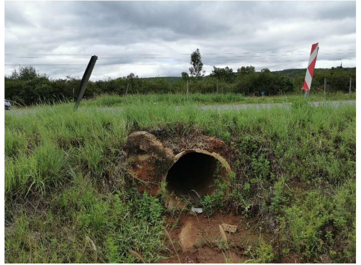
Dilapidated pipe culvert along the road
