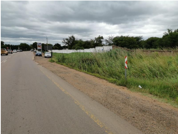
Poorly visible signage along the road to be revamped
