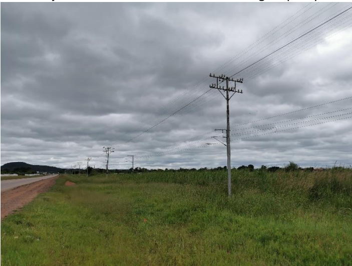
Electrical line parallel to the road in Bela Bela
